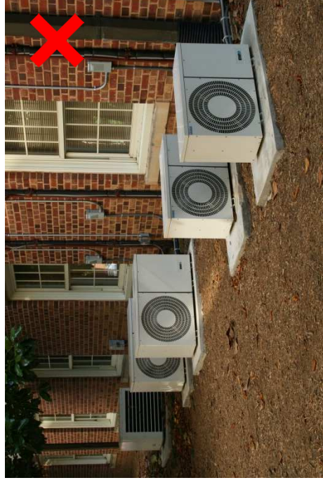
Inappropriately sited air conditioning units that are visually intrusive.
