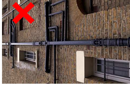
Drain pipes that ruin the buildings facade.
